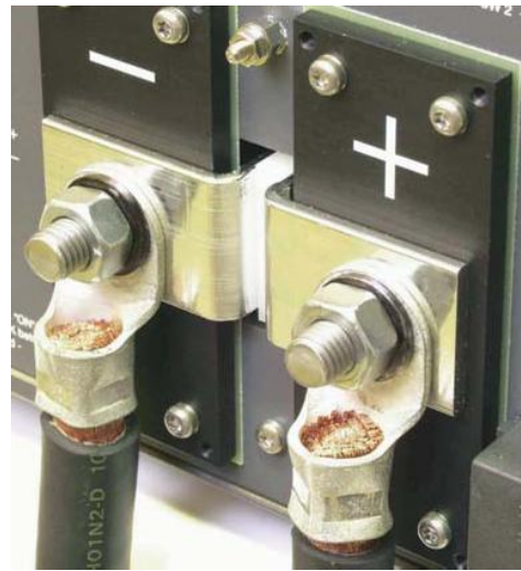
fig. 4 - 1 low resistive cable connection by mounting the cables directly on the tinned output strips
